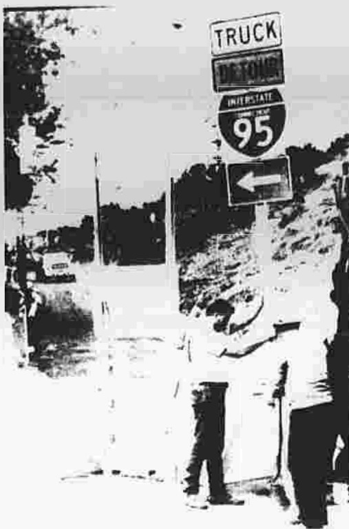
Traffic sign is erected on Strickland Road in Greenwich detouring truck traffic down temporary ramp away from the Mianus River Bridge.
